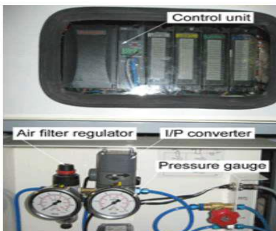
Fig. 3 Control unit and pressure system
